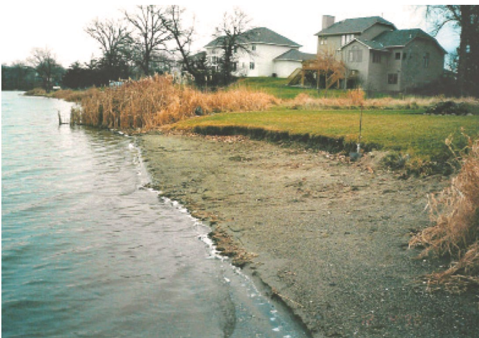
Erosion may be accelerated by activities such as boat wakes or high waves during storms. Each year erosion causes the loss of valuable shorefront property. Contrast the eroded shoreline lacking vegetation (foreground of photo) with the well-vegetated, uneroded shoreline in the distance.
