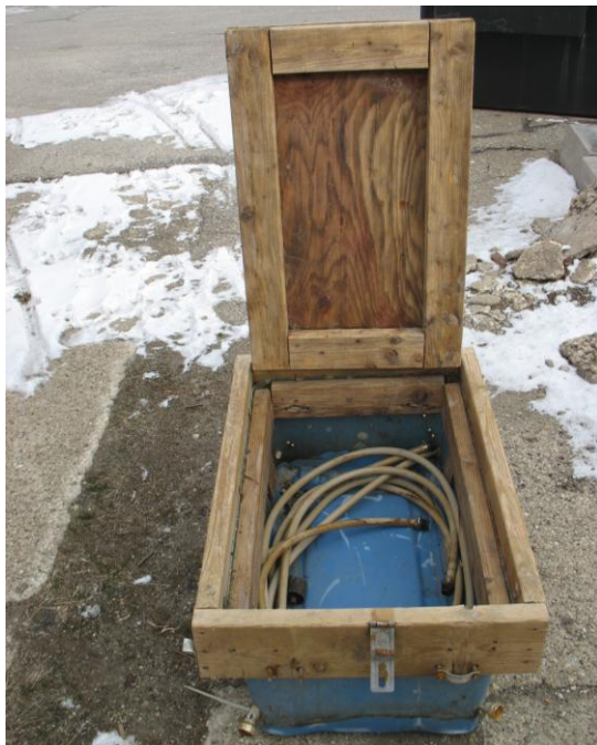
Figure 22: Pokegama Lake groundwater collection box.
